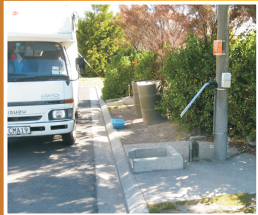
Campervan Discharge Point
