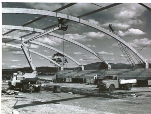
The Rotorua Sportsdrome under construction in 1963/64. At the time these were the largest laminated timber beams ever built in New Zealand. Rotorua Museum of Art and History, Te Whare Taonga o Te Arawa, OP 4724
