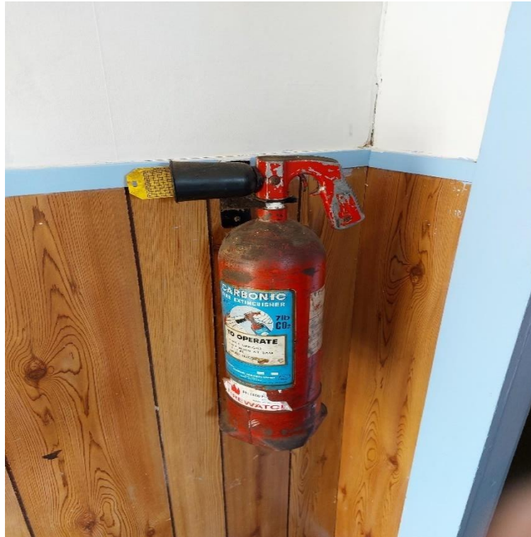
Image 18: Fire extinguishers on the wall in the escape route.
