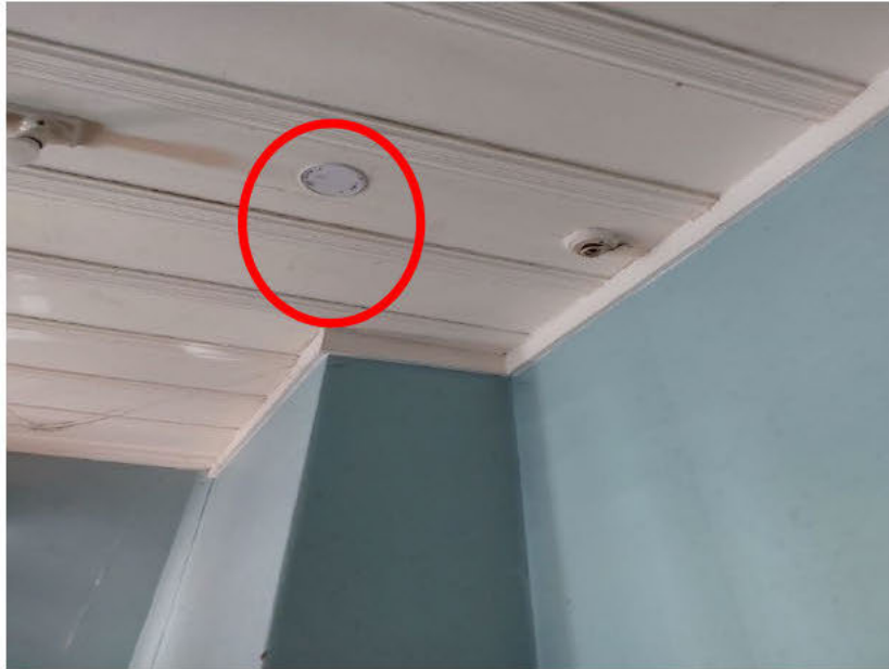
Image 14: Smoke alarm plate with smoke alarm removed.
