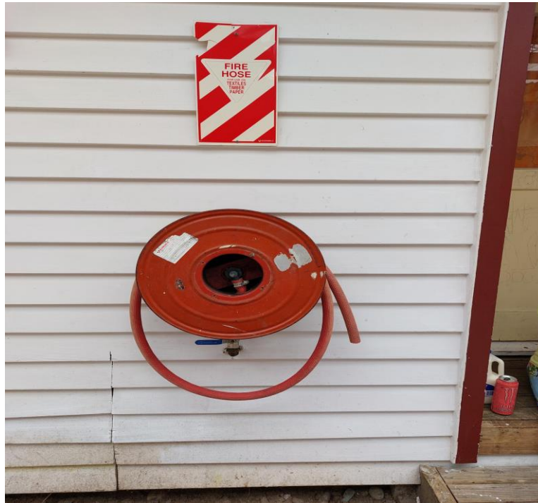
Image 21: Second fire hose located in the courtyard.
