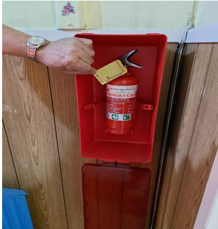
Image 19: Fire extinguisher near manager's office
