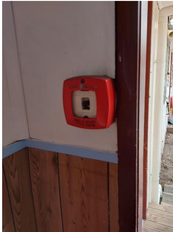
Image 22: Fire Action notice needs to be above all manual call points.
