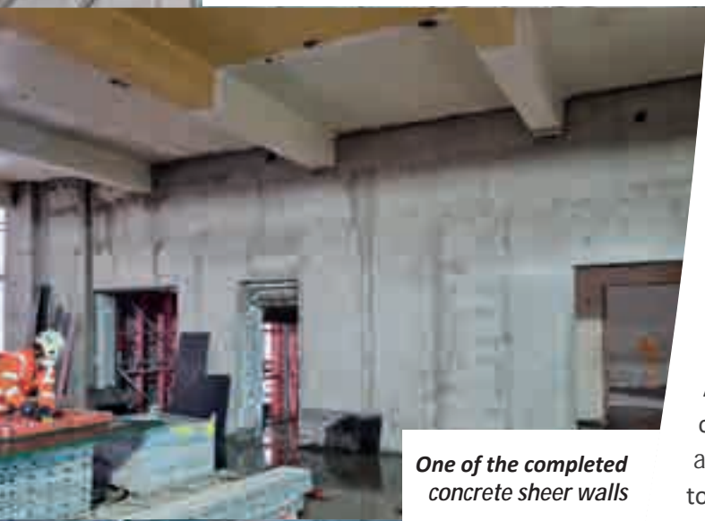
Concrete panels in place in the Concert Chamber, restored heritage trusses visible in the ceiling
