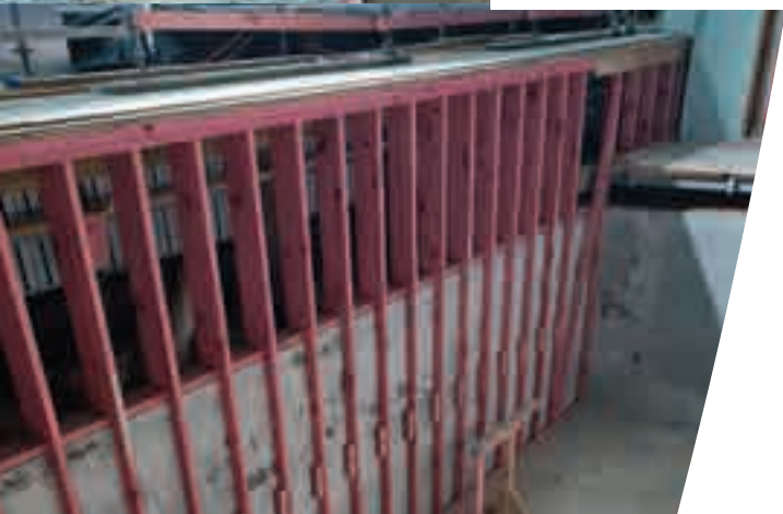
Finished orchestra pit in the Civic Theatre, ready for the lift to be installed
