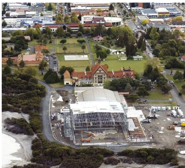
The new Energy Events Centre taking shape behind the Museum of Art and History in Government Gardens
