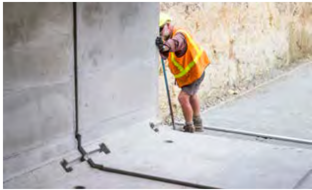
FIG. 6 Place the next culvert as close as possible to desired position and then pull into correct position with a come-along, connected to the swiftlifts in the culvert. Line up two half dog-bone connector recesses.
