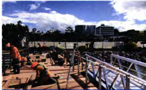
Tonka decking will be laid out and secured on the Lakefront boardwalk – similar to Access to Water shown here.
