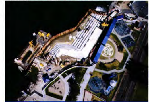
We will construct a coffer dam around the work area at the Lakefront similar to that used for Access to Water.
