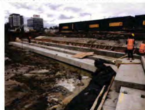
Terraces will be constructed within the coffer dams – similar to the process shown here during the Access to Water project.
