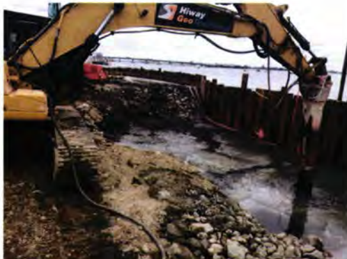
Ground improvements / cement stabilisation at Access to Water using digger and mixing arm attachment.
