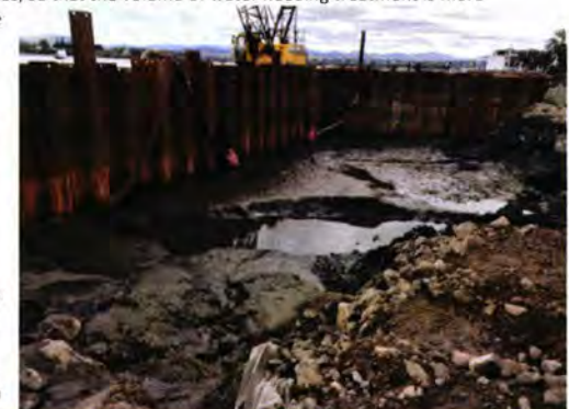
Dewatering pumps in progress on HEB's Access to Water project. For Rotorua Lakefront we will pump the lake water out into treatment tanks before discharging.
