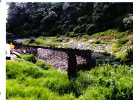
Environmental protection is paramount in HEB's current Waiani Water Intake Scheme where we have diverted the stream to rebuild the existing stream bed. We will take the same care when working in the Rotorua Lake edge.
