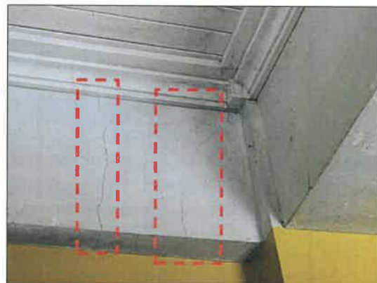
(f) Men bathroom – Cracks across the beam
