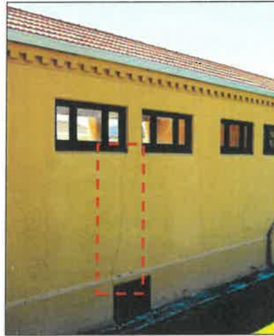
(h) Men bathroom – Cracks across the beam
