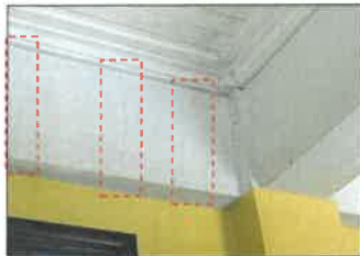
(h) Flexural cracks along the beam supporting roof structure
