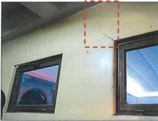
(g) Storage room on the right-hand side of the pool – Cracks across the wall
