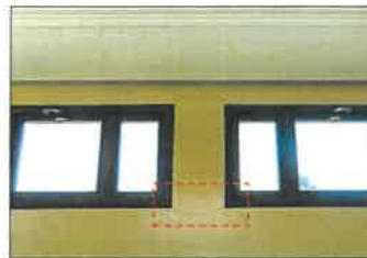
(i) Cracks between opening – Short column phenomenon
