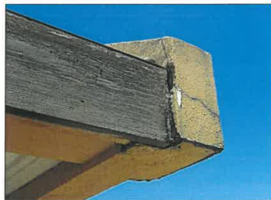
(l) Office on the first floor – Deteriorated connection at the office roof corner
