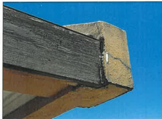
(l) Office on the first floor – Deteriorated connection at the office roof corner
