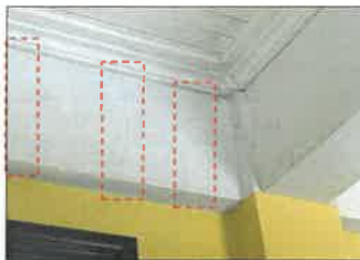
(h) Flexural cracks along the beam supporting roof structure
