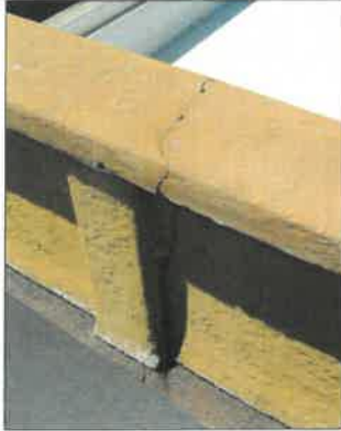
(f) Parapet showing cracks from first floor terrace
