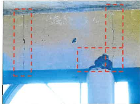
(j) Storage room on the left-hand side of the pool – Cracks across the beam and deteriorated connection between the column and the beam
