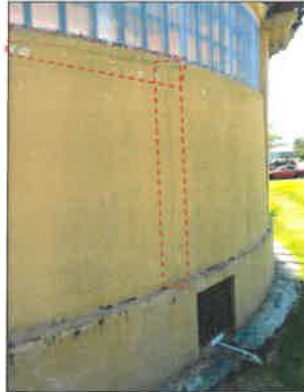
(g) Cracks along and across outside wall at southern wing
