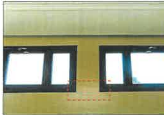
(i) Cracks between opening – Short column phenomenon
