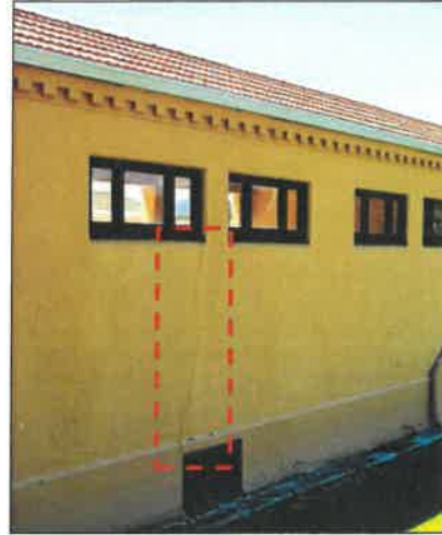
(h) Men bathroom – Cracks across the beam
