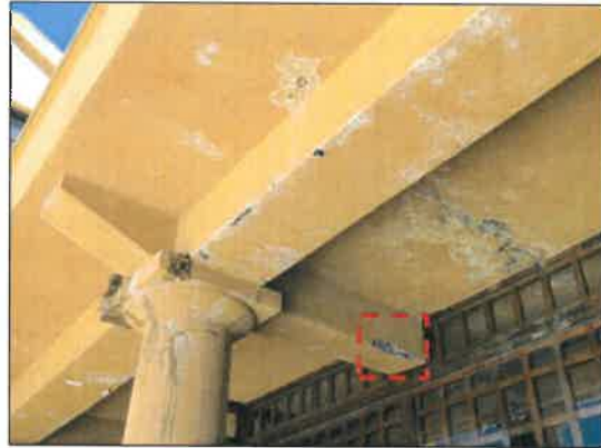
(b) Underneath the first-floor terrace – Spalling of the beam
