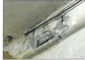
(j) Spalling of a RC beam with rusted reinforcements
