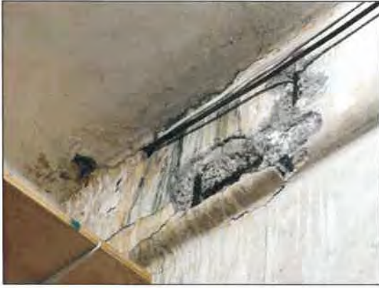
(m) Room within a courtyard area - Spalling of a RC beam with rusted reinforcements
