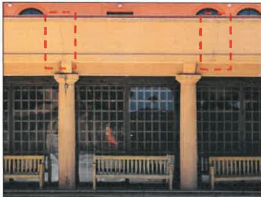
(a) Walkway next to the pool – Cracks across the parapet
