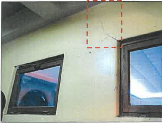
(g) Storage room on the right-hand side of the pool – Cracks across the wall
