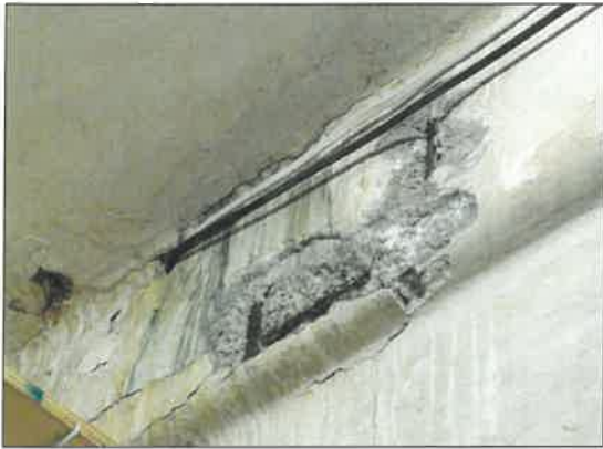
(t) Spalling of a RC beam with rusted reinforcements
