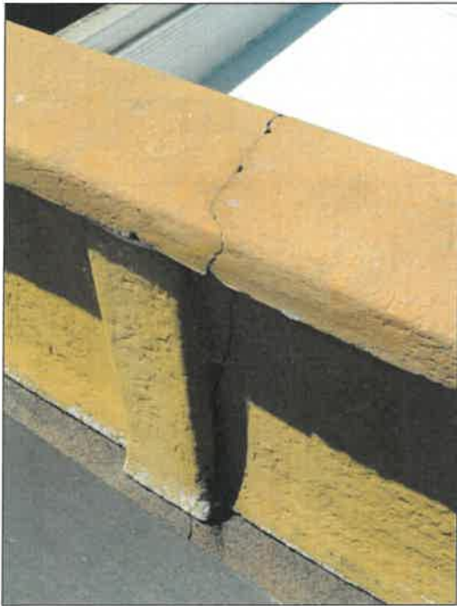
(v) Same parapet showing cracks from first floor terrace
