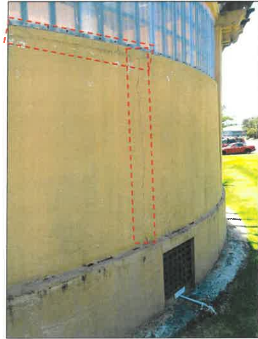
(w) Cracks along and across outside wall at southern wing
