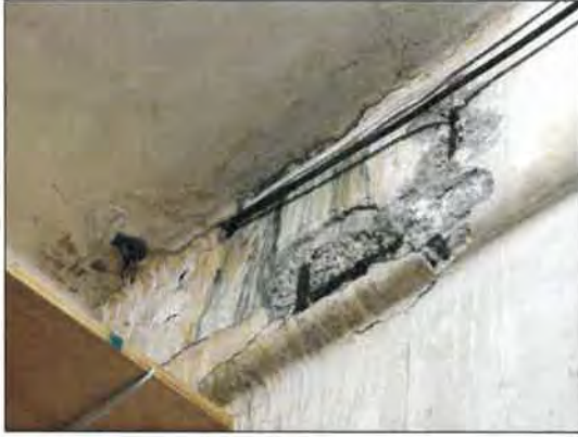
(m) Room within a courtyard area - Spalling of a RC beam with rusted reinforcements
