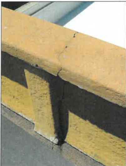
(k) First floor terrace – Cracks across the parapet
