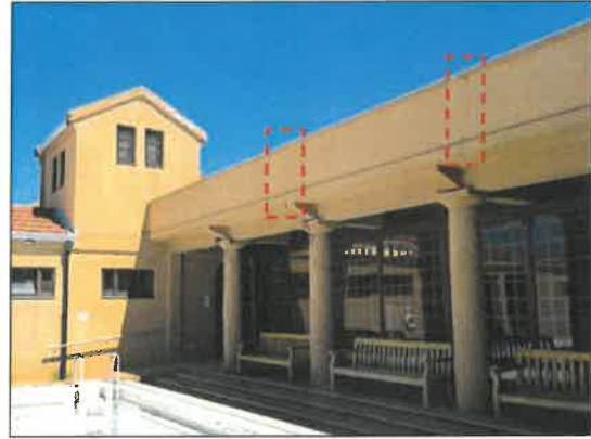
(u) Cracks across the parapet facing the pool
