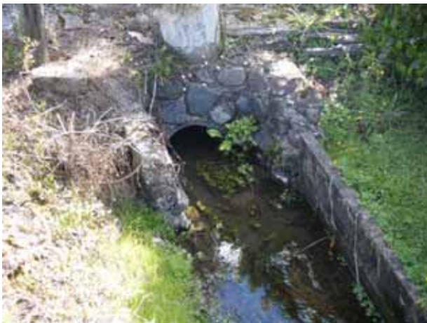
Figure 20: Potential artificial barrier (culvert) to fish passage observed within Benn Road Stream.
