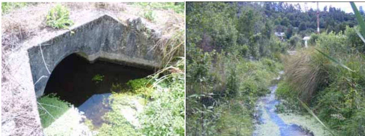
Figure 9: DP6 and 7, the discharge point to Lake Okareka. The photo on the left shows the pipe outlet to an open channel/drain that flows to the lake. The drain is shown in the photo to the right looking from the lake edge.
