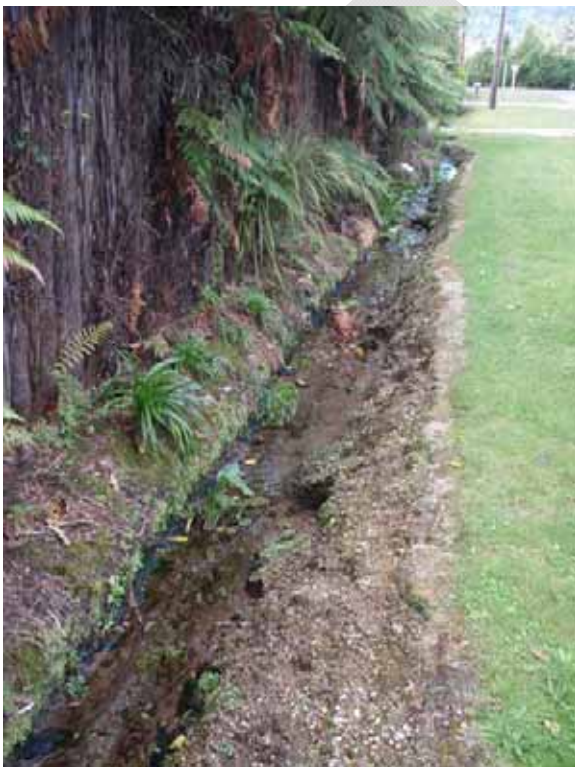
Figure 15: Benn Road open drain and minor erosion of main channel.
