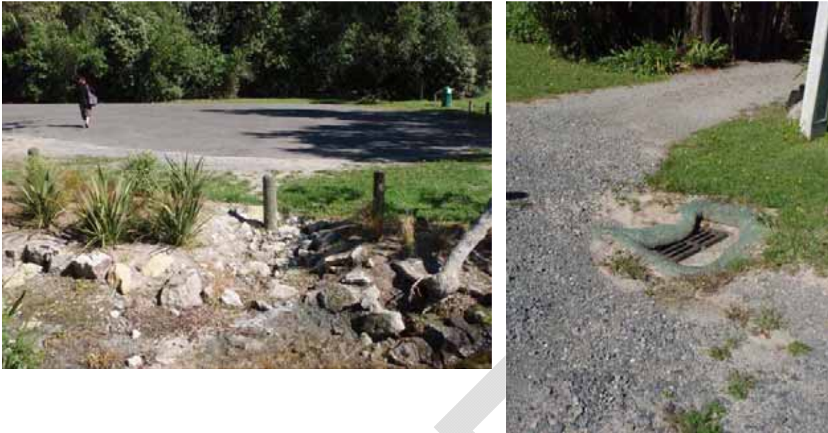
Figure 12: Left – Turnaround point with a discharge to lake. Sediment on road margins drain to lake without treatment. Right – Gravel driveway next to catchpit with silt/gravel diversion bags around grate.
