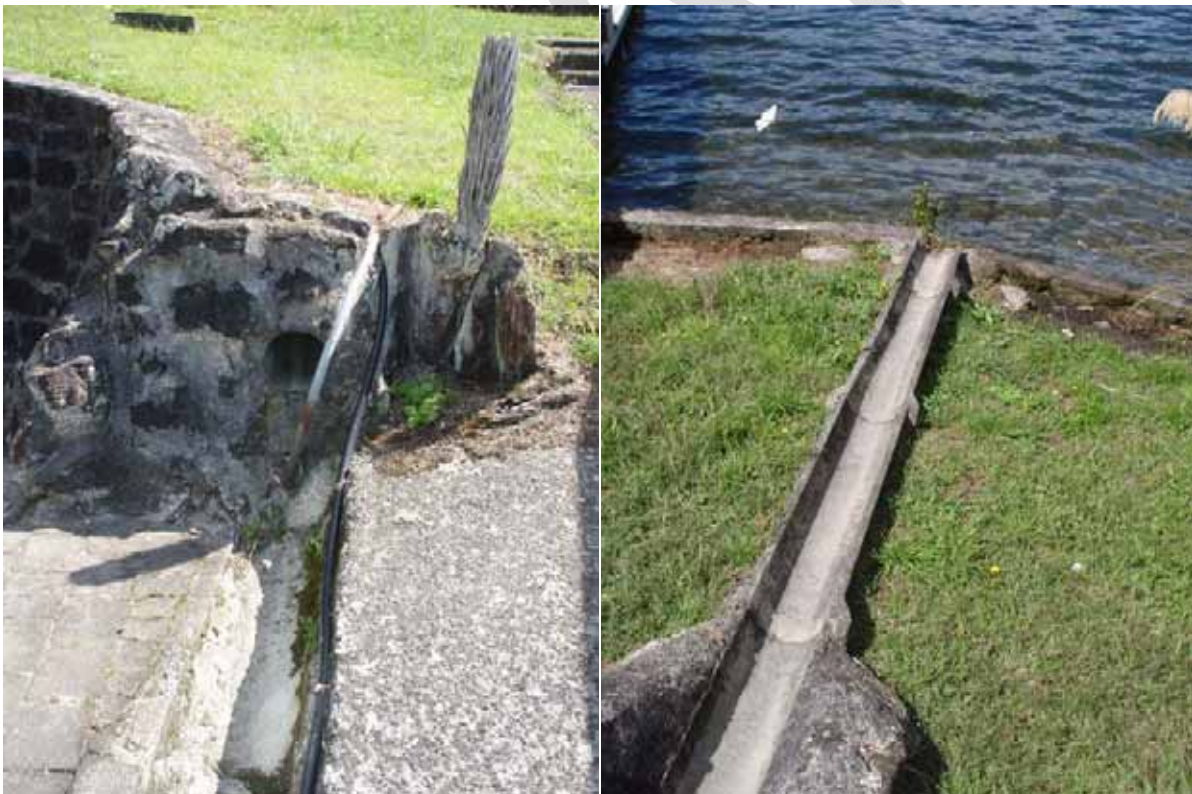
Figure 7: DP4, the discharge point to Lake Okareka. The photo on the left shows the pipe outlet to a small open channel that spills to the lake as shown in the photo to the right.
