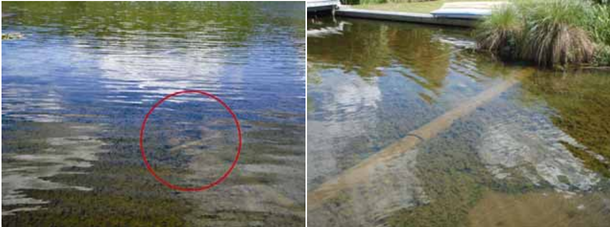
Figure 11: DP9 discharge point on the edge of Lake Okareka. The photo to the left shows the submerged pipe end and the photo on the right shows the submerged pipe leaving landfall.
