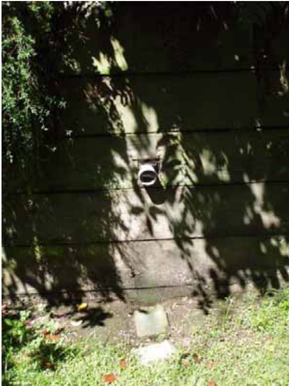
Figure 14: Minor erosion around a private stormwater connection pipe flowing into The Wash and the rudimentary measures to control erosion.
