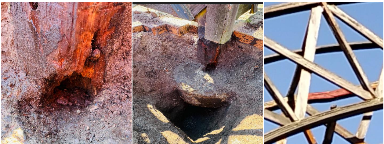
Figure 2,3,4: Decay of post in contact with in-situ soils; exposed 600 x 220mm concrete footing; & damaged top chord.
