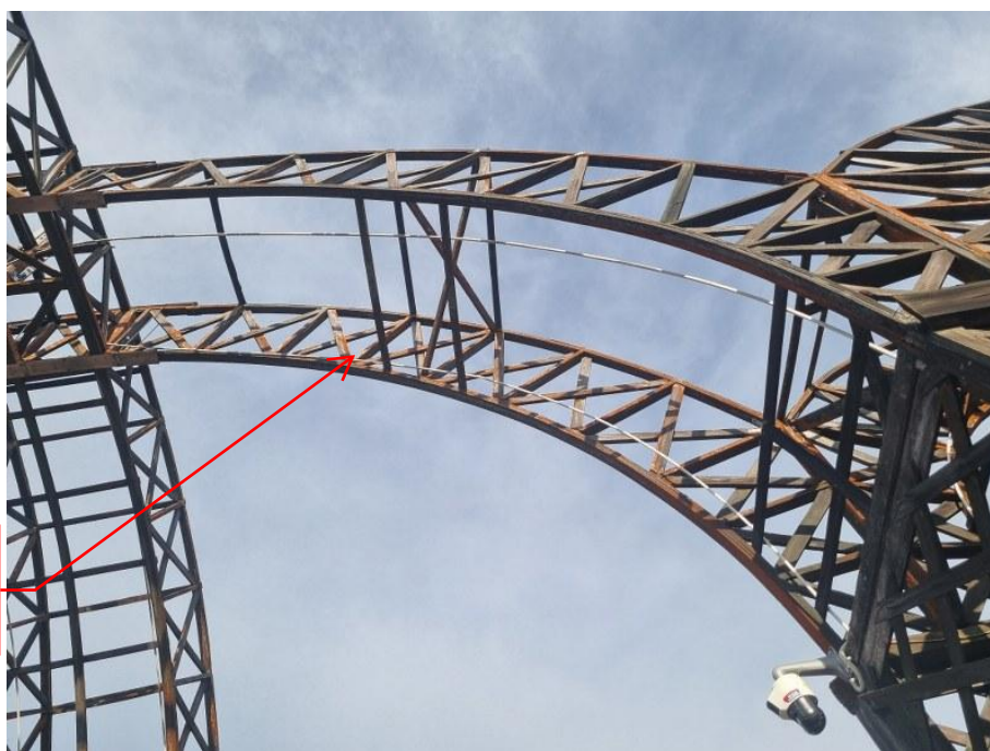
Figure 4: North-West Primary Arch Span showing missing members between top and bottom chords Adjacent spans shown the original density of framing
