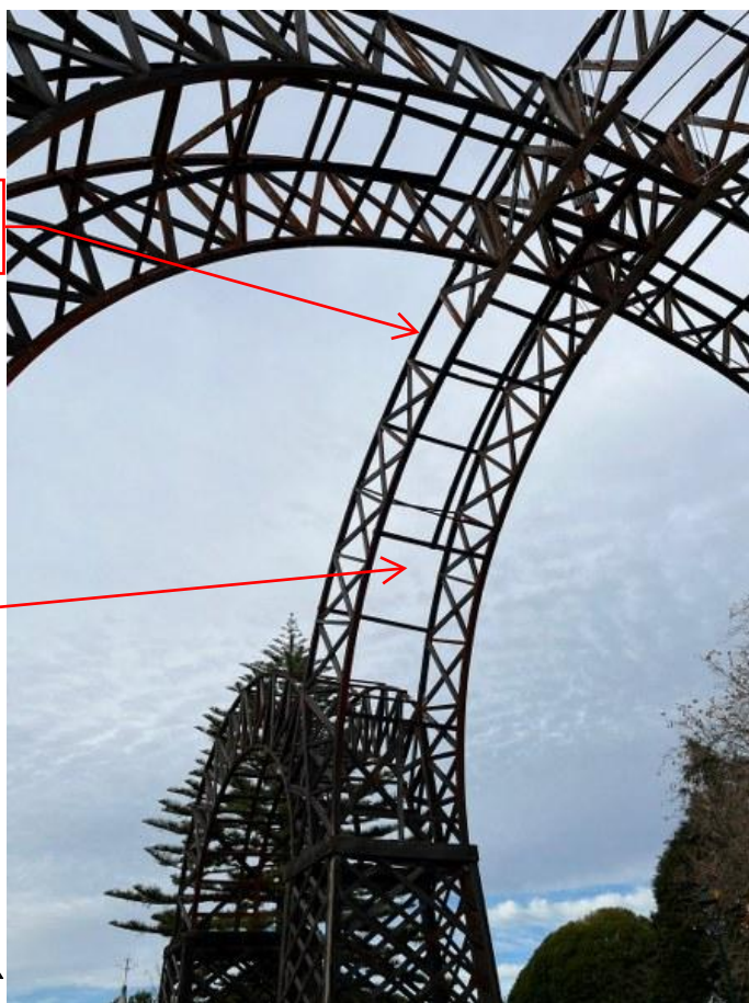
Figure 5: South-East Primary Arch Span showing missing members between top and bottom chords Adjacent spans shown the original density of framing, Diagonal Bracing missing second bay from apex.
