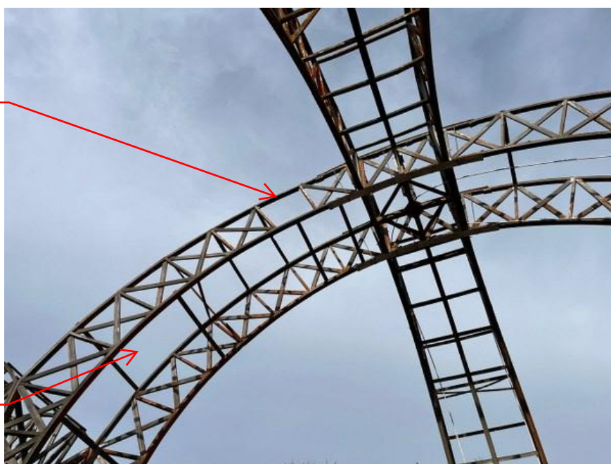
Figure 6: South-East Primary Arch Span showing missing members between top & bottom chords Adjacent spans shown the original density of framing, Diagonal Bracing missing second bay from apex
