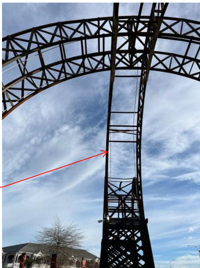
Figure 3: North-West Primary Arch Span showing missing members between top & bottom chords Adjacent spans shown the original density of framing
