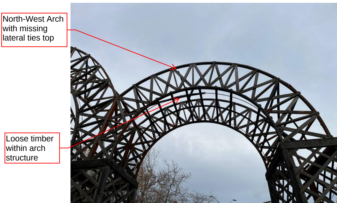
Figure 7: North-West Secondary Arch Span showing missing members to top chord, note timber laying within arch
