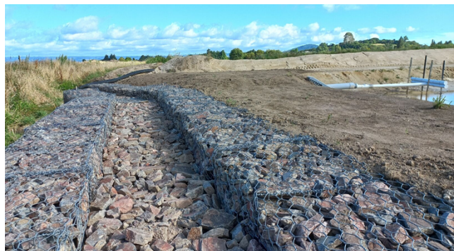
Mansfield Road Subdivision – stormwater swale
