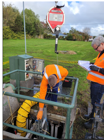
Above: TRILITY staff working at pump station at Nqonqotaha
