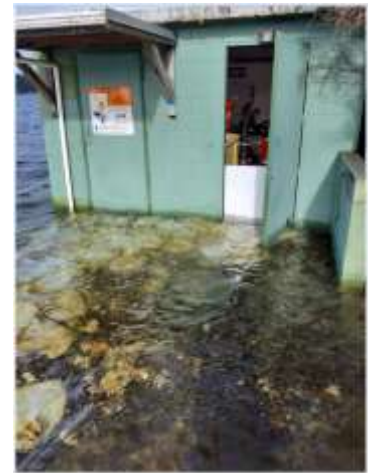
Current water level at Rotomā wastewater treatment plant
